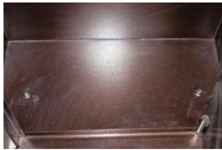
With the bolts seated in their holes, it is a simple matter to fasten them firmly with a spanner or socket wrench. The job is almost complete!
